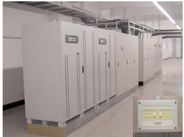
One of the parallel 250kVA Master Dialog UPS Systems and the USG accessory
