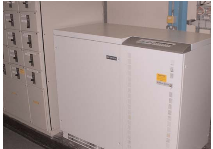
The 30kVA MasterDialog UPS for the air filtration plant
