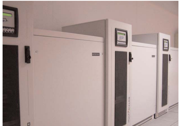
The Multi Dialog 60kVA Systems At ING Direct Cardiff
